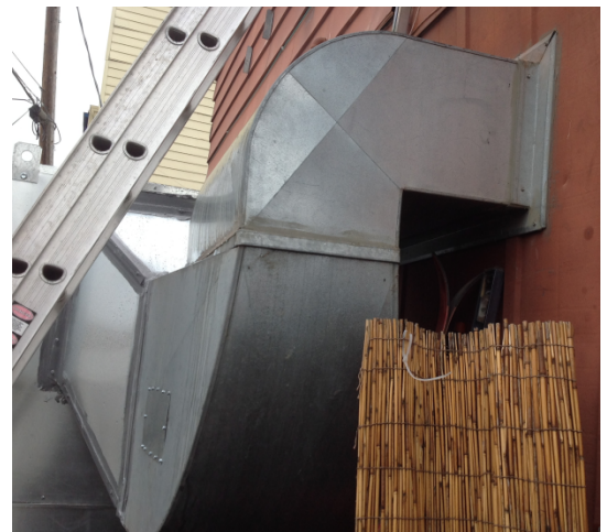
Figure 2: Poor duct install
