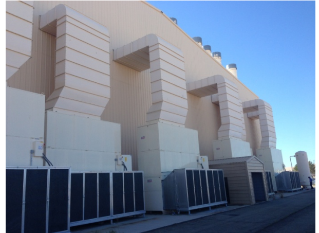
Figure 1: Good duct install
